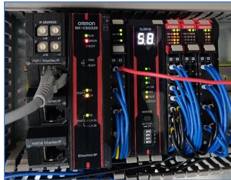
Figure 5. Omron Safety PLC
