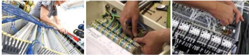
Figure 1 - Typical switchgear wiring operations
