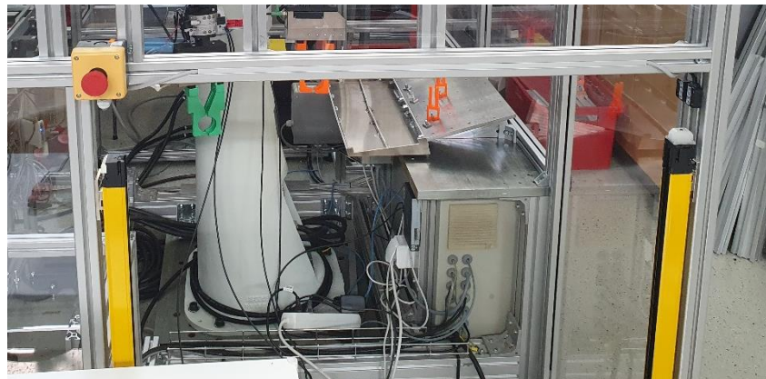
Figure 28. Safety devices: Emergency stop buttons, light curtains, and a door switch.
